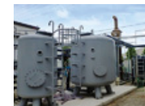
Grey water facilities (Soka Factory)
