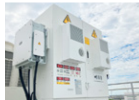
Lithium-ion battery (Soka Factory)
